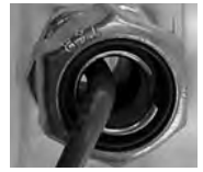
Conduit with Cable
